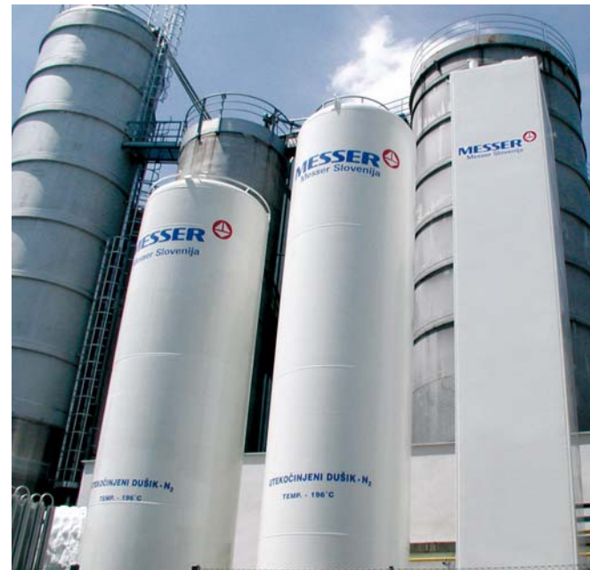
The Messer Group's smallest air separator was installed at Julon.
