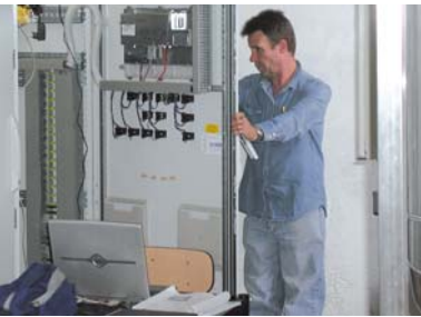
Brennand Hall, Project Manager Engineering and Production, during installation work in Slovenia.
