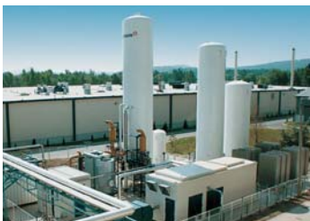
A second nitrogen generator was commissioned at Zoltek.
