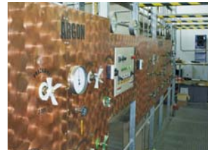
New filling points are making the plant at Police more productive.
