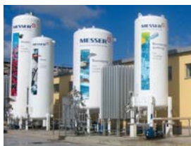
The new headquarters of Messer Chimco Gas has its own filling facility.
