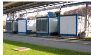
Membrane plant – nitrogen delivery for on-site customers OKD, DPB.
