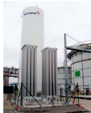
Waste water treatment plant Spolchemie in Usti nad Labem.
