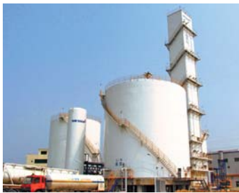
An air separation plant also came on stream in Zhangjiagang.
