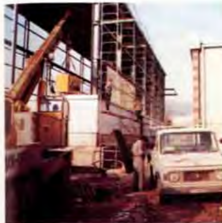
Erection of refrigeration circuit compressor for new air separation plant in Austria
